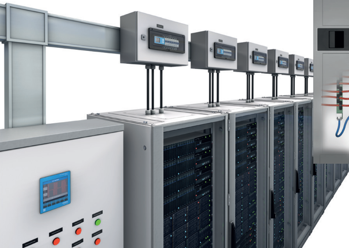
Tap Off monitoring in bus way systems
